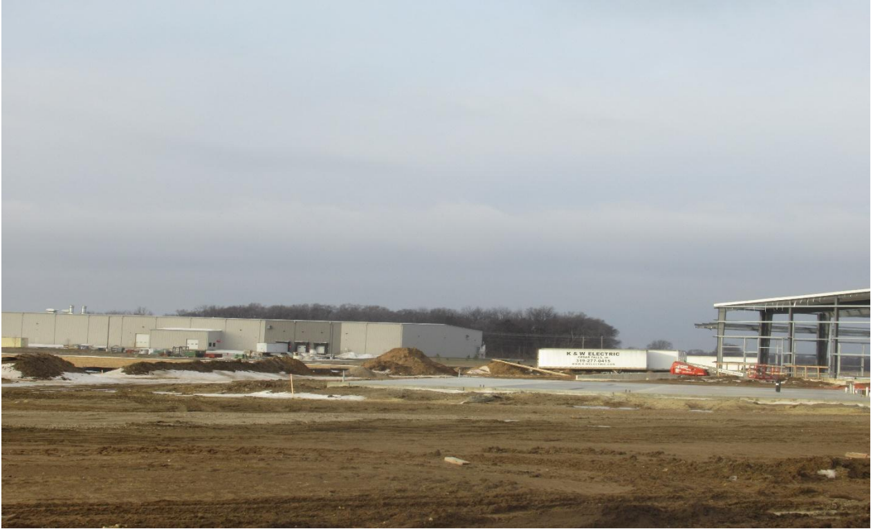
Picture 2: Looking southwest from Warp Drive with the new expansion to the right of the existing building.
