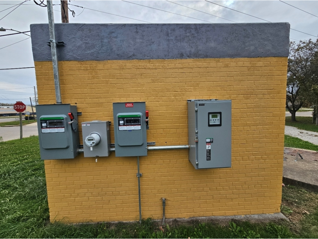
New hookup for portable generator and a manual transfer switch
