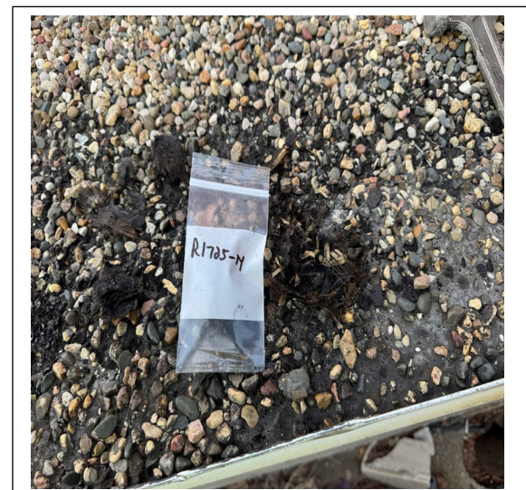
Sample R1925-14: Flashing from lower NW roof positive for asbestos.
