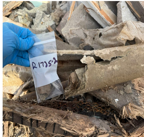
Sample R1725-2: Pipe insulation from West building in demolished part of building positive for asbestos
