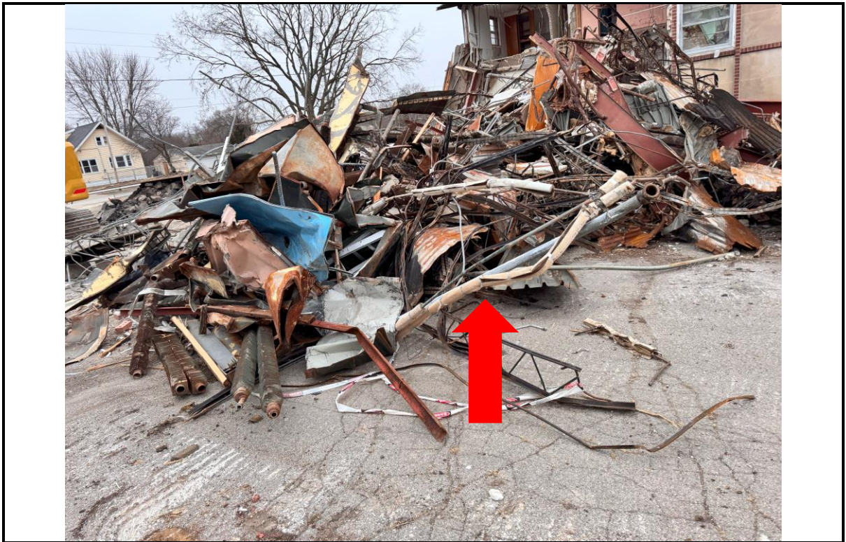
Photo 5: View of asbestos TSI piping in scrap pile on the east side of the Villa.
