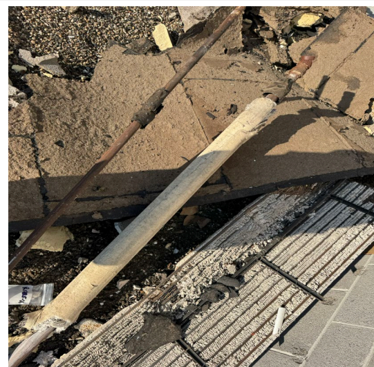
Mag pipe from SW addition of the larger building positive for asbestos.
