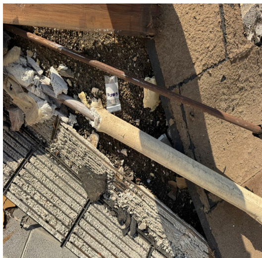
Sample R1925-21: Mag pipe from SW addition of the larger building positive for asbestos.
