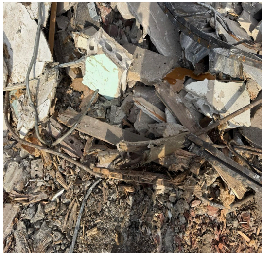
Pipe insulation found in debris pile.
