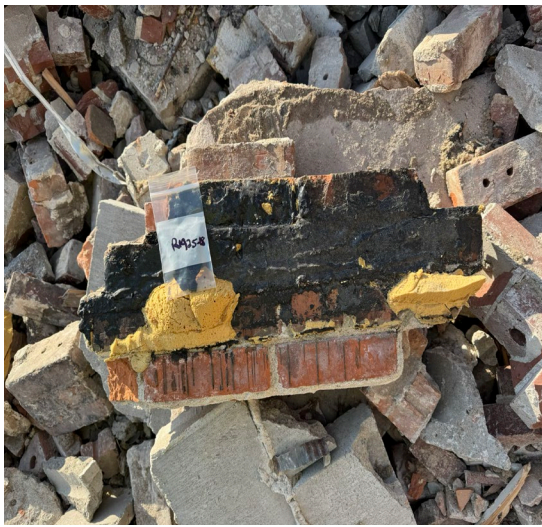
Sample R1925-18: Tar on brick in SE debris pile positive for asbestos. (Believed to be from upper parapet wall, but unsure). Only one small section of brick found.
