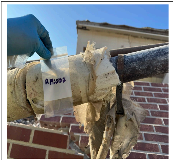
Sample R1925-22: Mag pipe in SW addition of larger building positive for asbestos.
