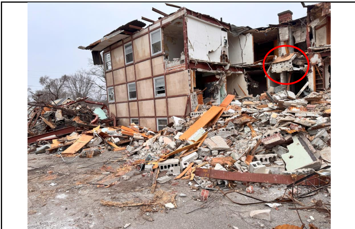
Photo 3: View looking at the debris pile on the east side of the Villa. Red circle showing suspect wall panel adhesive that was not sampled.
