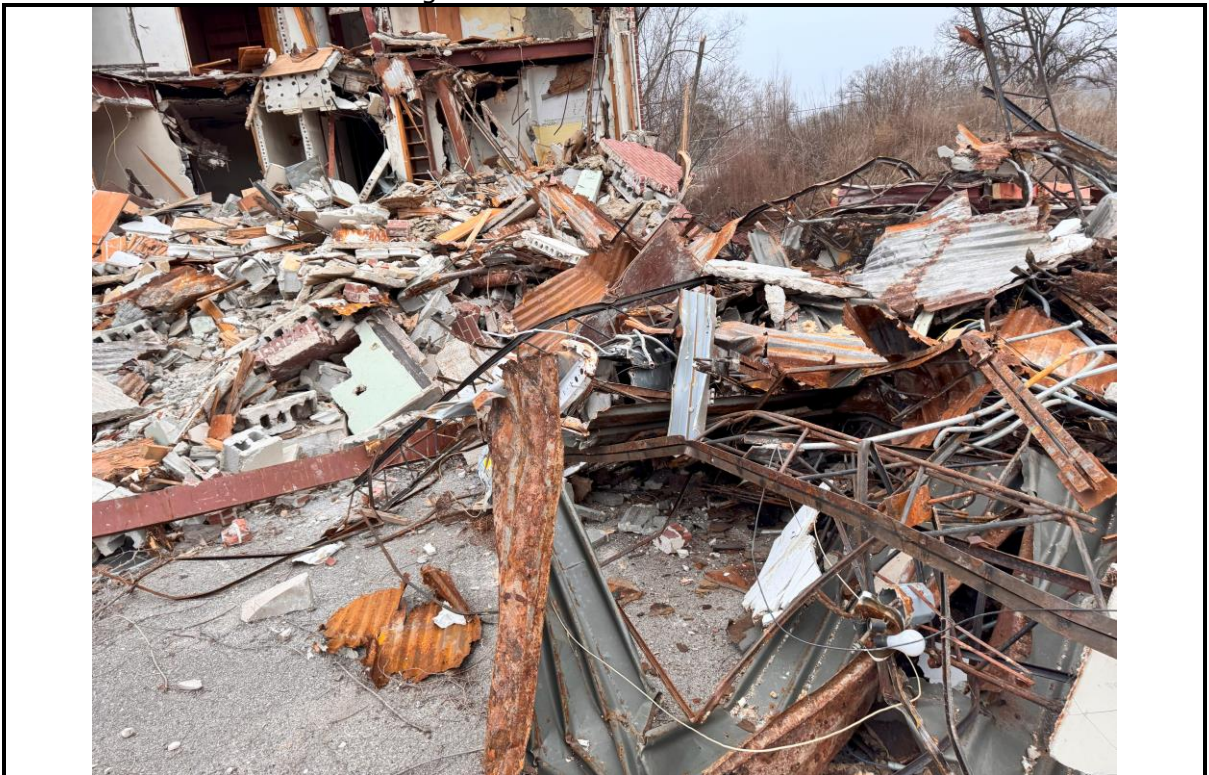
Photo 8: View of the rubble pile on the northeast corner of the building.
