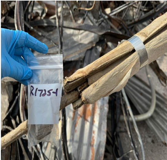
Sample R1725-1: West building pipe insulation from demolished portion of building positive for asbestos.
