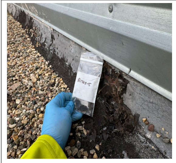
Sample R1925-15: Flashing from lower NW roof, larger building, positive for asbestos.
