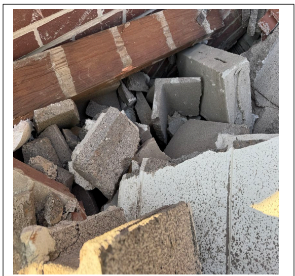
Mag pipe in debris pile SW addition of larger building.
