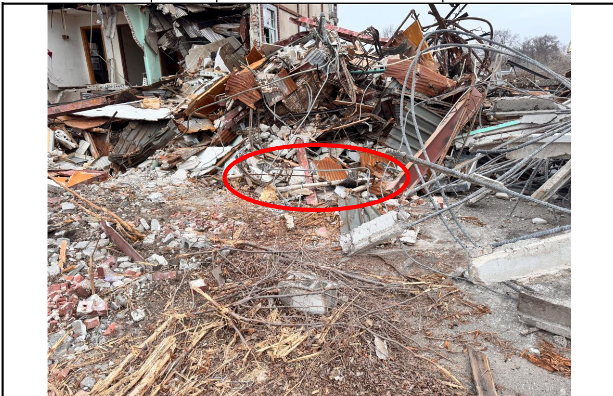
Photo 4: View of asbestos containing thermal systems insulation (TSI) piping in debris pile.
