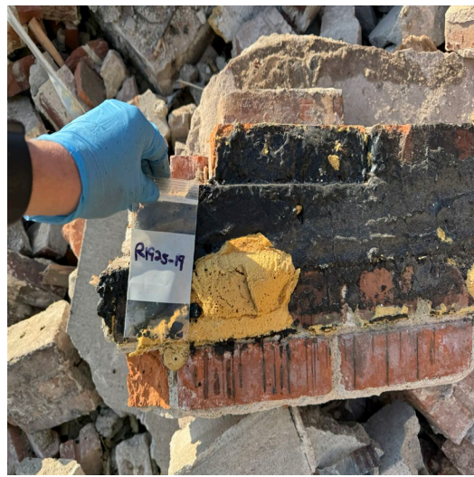
Sample R1925-19: Tar on brick in SE debris pile positive for asbestos. (Believed to be from upper parapet wall, but unsure). Only one small section of brick found.
