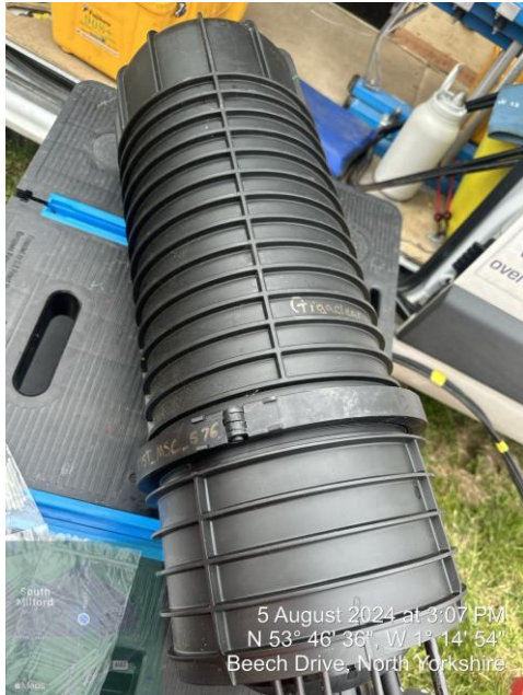
Documented Fiber Enclosure
