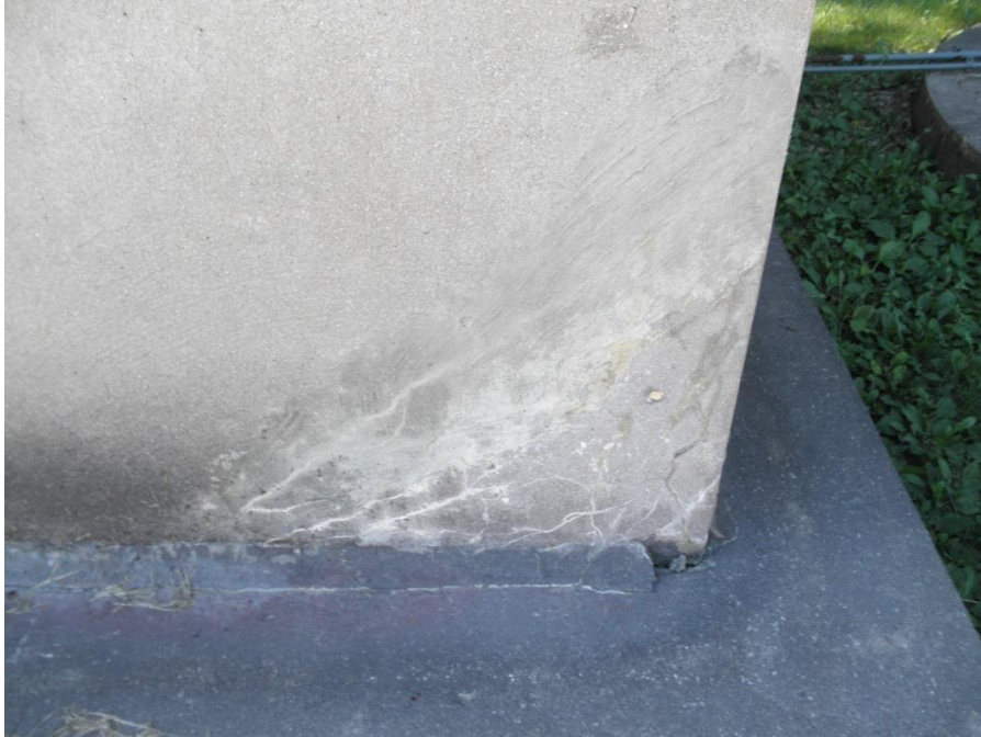
Picture T7: Cracked Dry Well Walls at Exterior Corner
