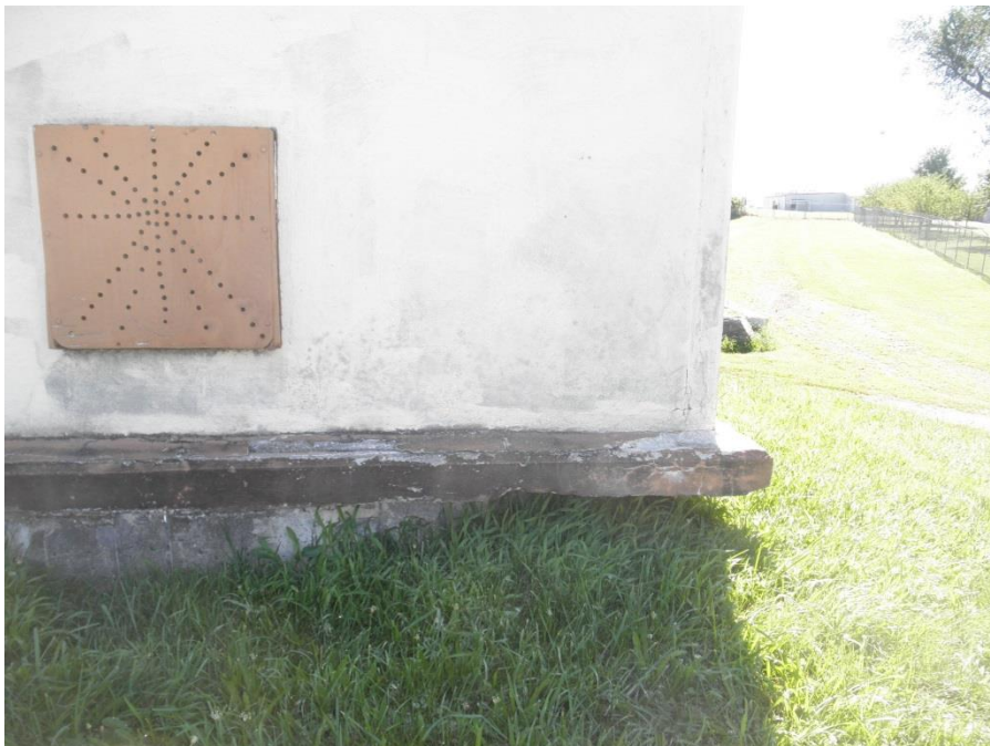
Picture CC8: Cracked/Spalled Exterior Slab and Lower Corner of Dry Well At-Grade Structure
