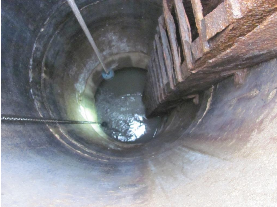
Picture CC5: Wet Well with Corroded Trash Basket
