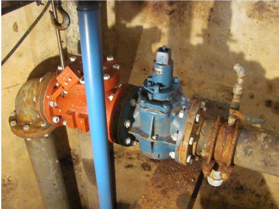
Picture NH8: Corrosion on Discharge Piping With Newer Check Valve
