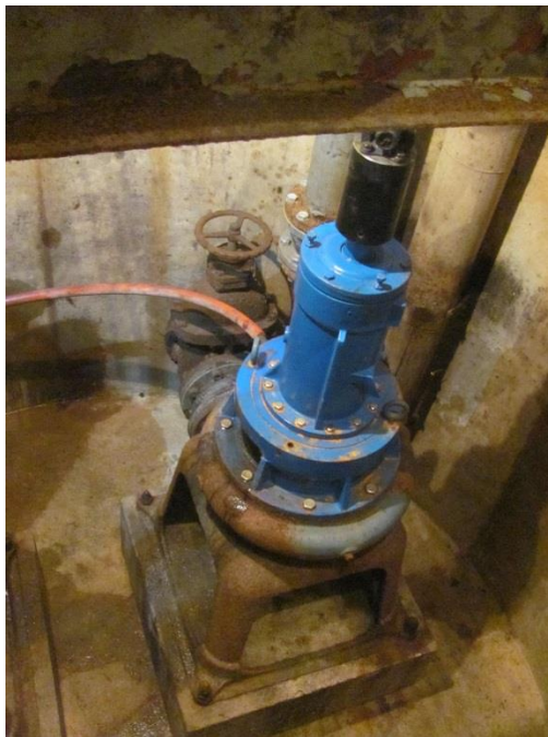
Picture NH9: Pump with Corroded Pump Base
