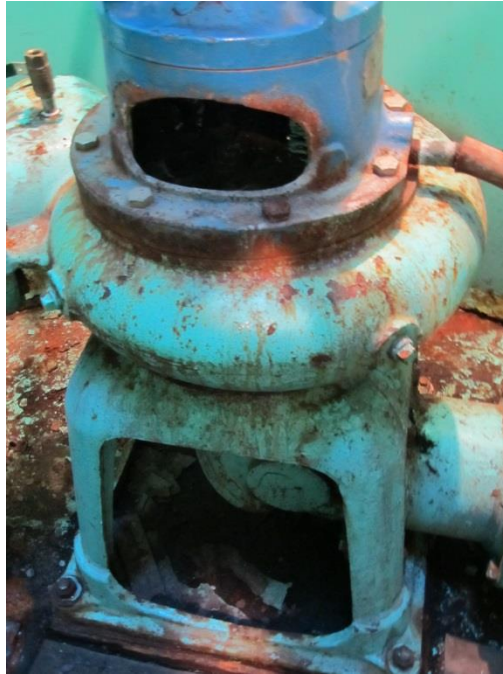
Picture H63S4: Light Corrosion of Pump
