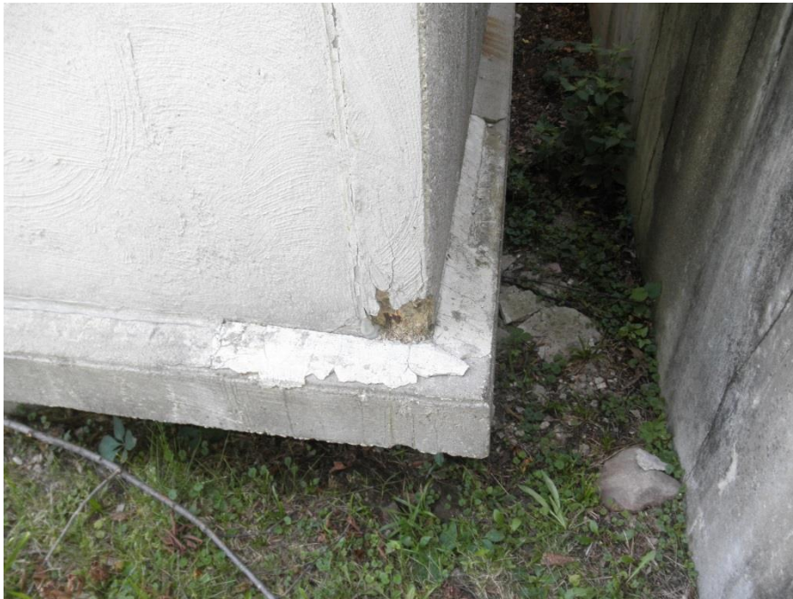
Picture NH13: Minor Spalling at Lower Corner of Wet Well Structure
