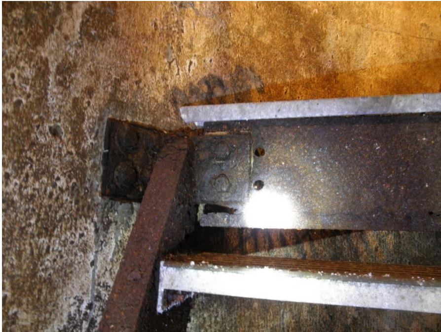
Picture CC11: Close-Up of Severely Corroded Channel Stairway Support
