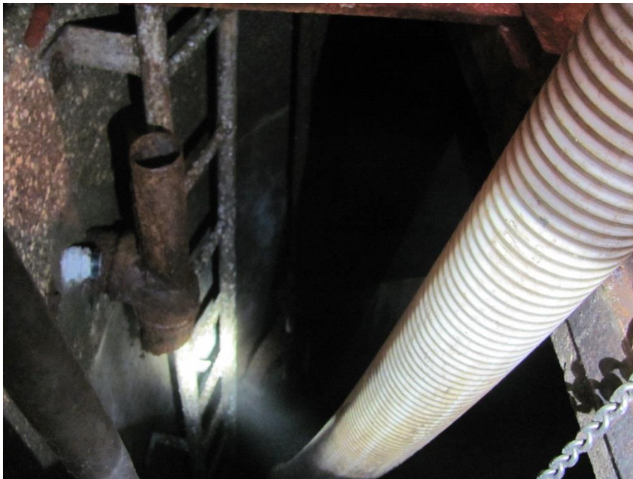
Picture NH11: Corroded Metal in Wet Well
