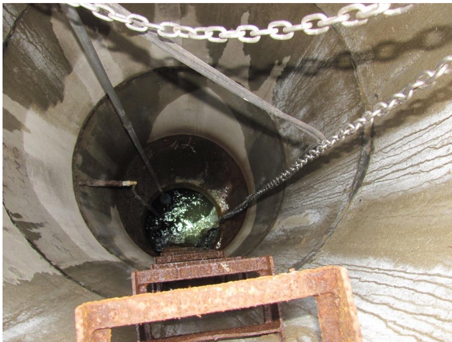
Picture H63S5: Wet Well Concrete (Typ.); Note Ladder Rung Corrosion
