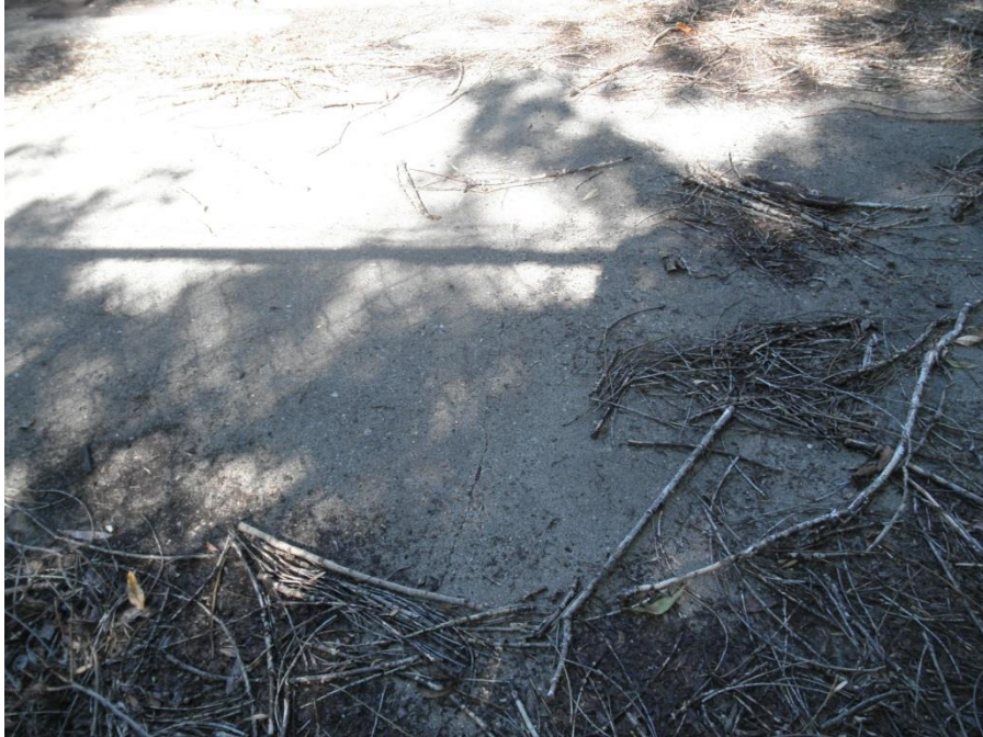
Picture NH6: Crack in Slab Topping
