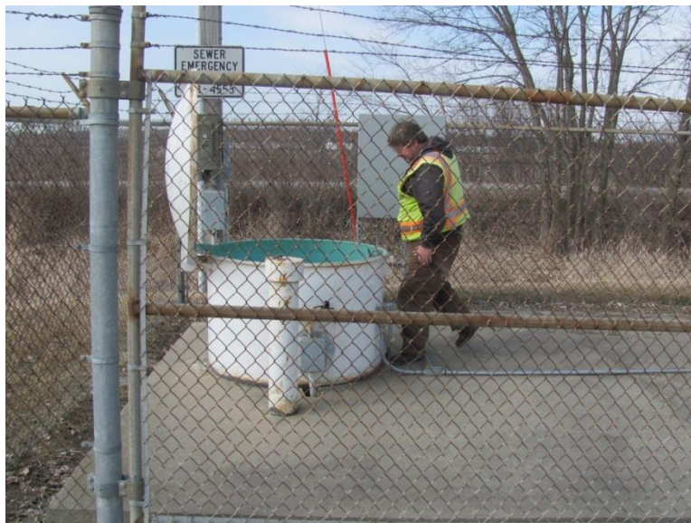
Picture H63S1: Hihgway 63 South Lift Station – Coated Steel “Can” Dry Pit on Grade
