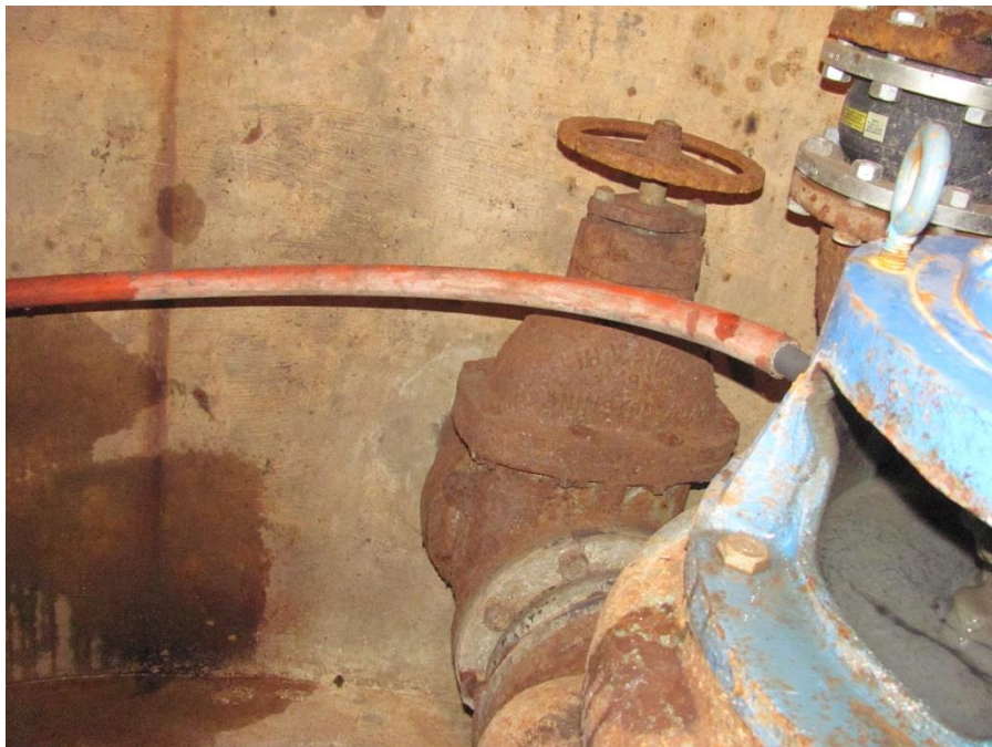
Picture NH7: Corrosion on Inlet Valve
