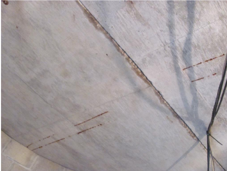
Picture NH12: Exposed Rebar in Dry Well Slab
