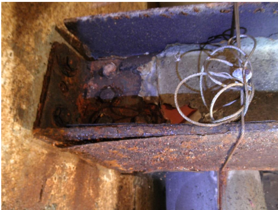
Picture CC12: Severely Corroded and Delaminated Structural Beams
