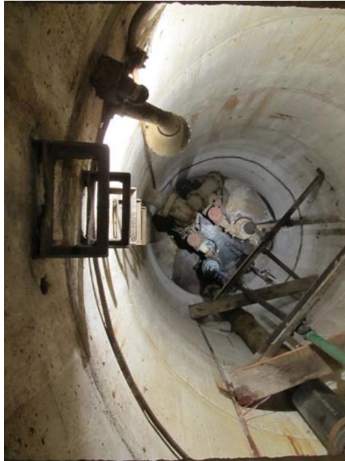
Picture T3: Overall View of the Pumps in the Dry Pit
