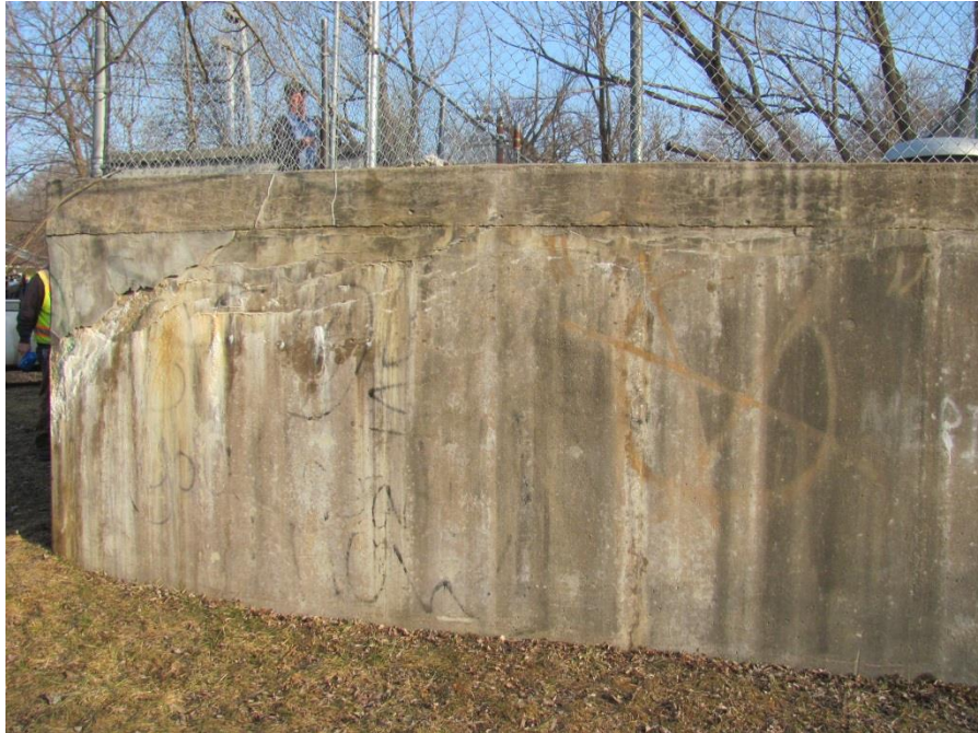
Picture NH4: Continued Deterioration Around Patched Corner Spall (Typ.)
