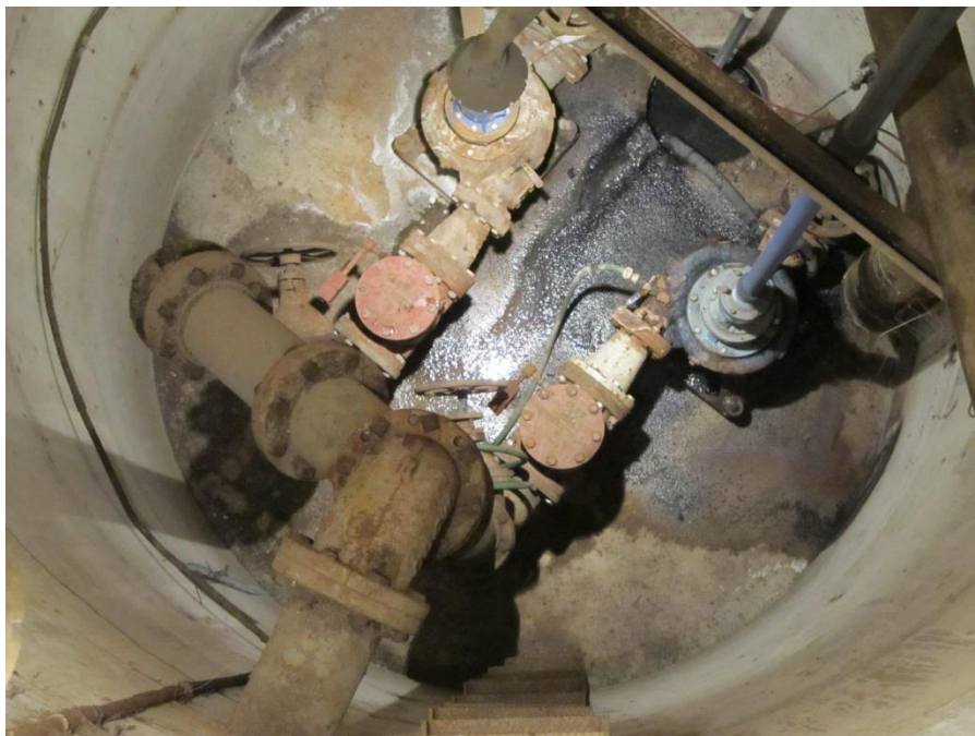
Picture T2: Pumps and Discharge Piping
