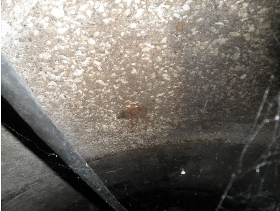
Picture NH10: Exposed Aggregate in Upper Wet Well
