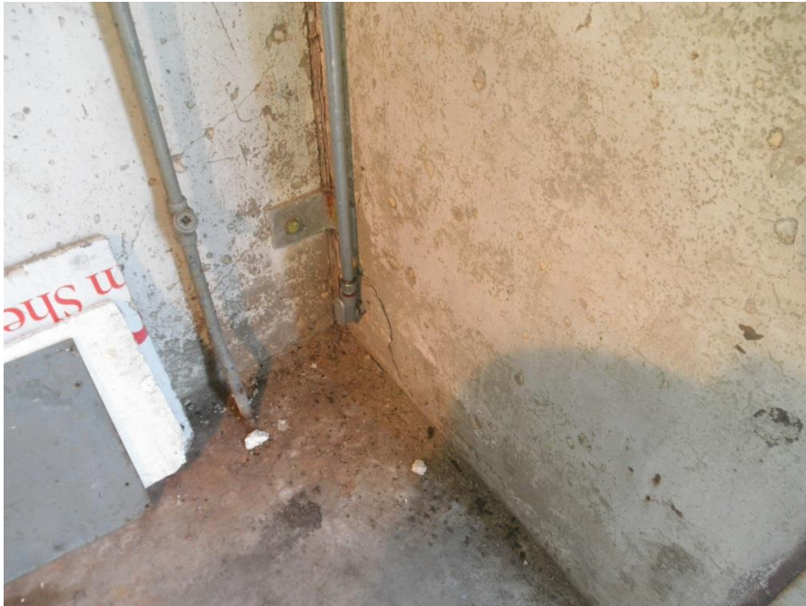
Picture CC7: Cracking at Lower Interior Corner of Dry Well At-Grade Structure
