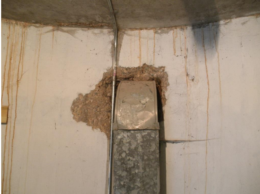
Picture D6: Spalled Concrete Around Vent
