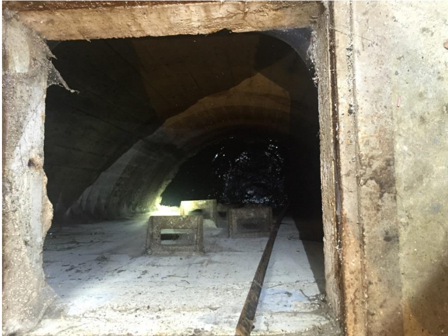
Picture D4: Wet Well
