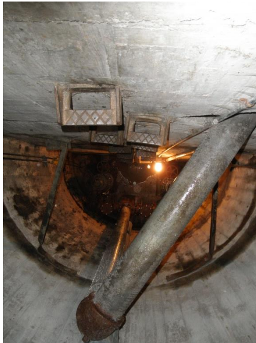
Picture D3: Dry Well Piping and Stairs
