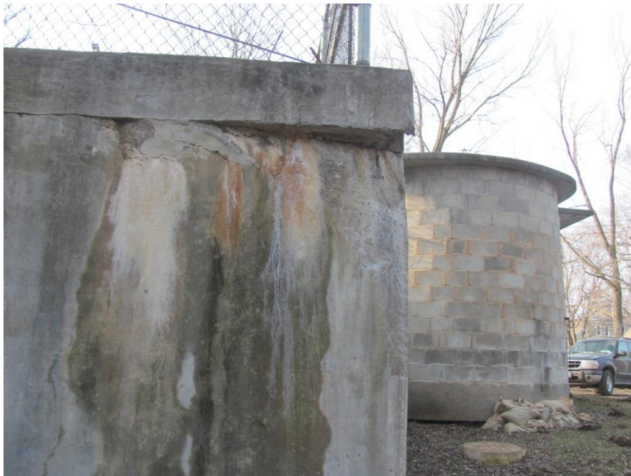
Picture NH3: Storage Tank Concrete Wall Deterioration at Top of Wall Corners (Typ.)
