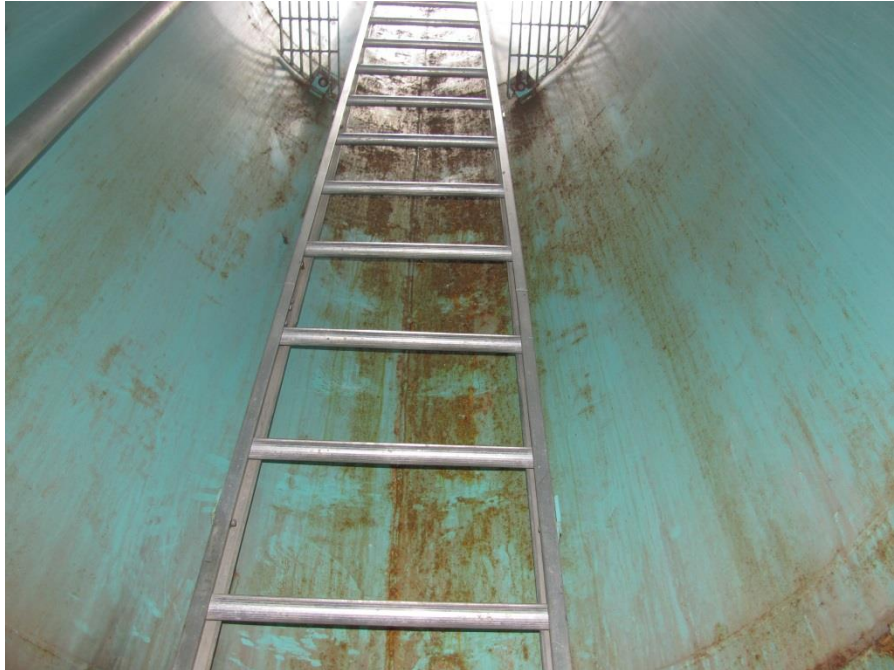
Picture H63S6: Light Corrosion of Dry "Can" Surface (Typ.)
