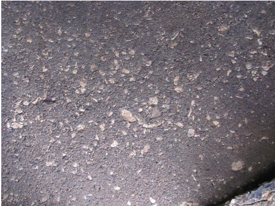
Picture CC4: Exposed Aggregate in Upper Wet Well Walls
