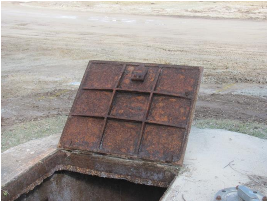
Picture T6: Corroded Wet Well Access Hatch
