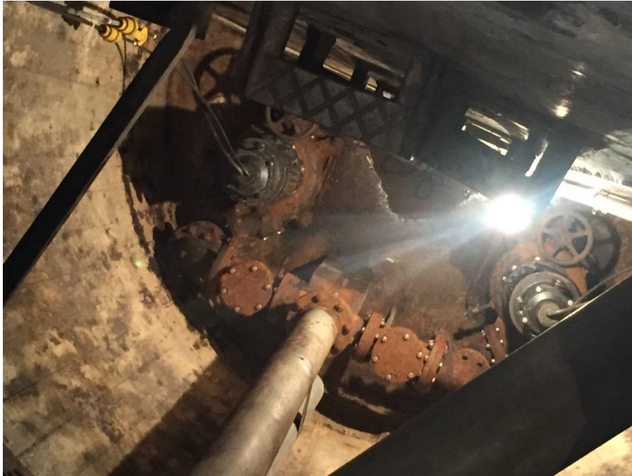
Picture D2: Light Corrosion of Pumps and Discharge Piping
