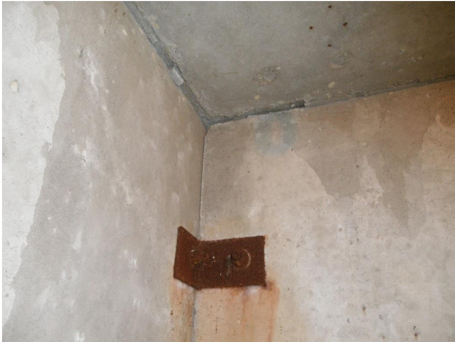
Picture T8: Corroded Wall Bracket of Dry Well At-Grade Structure
