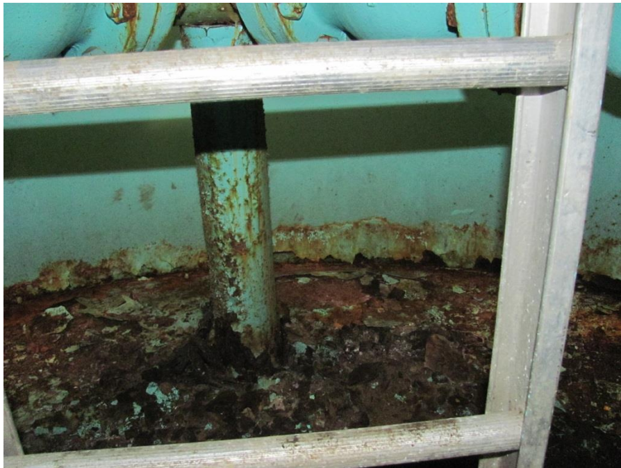
Picture H63S7: Corrosion at the Bottom of the Dry "Can"
