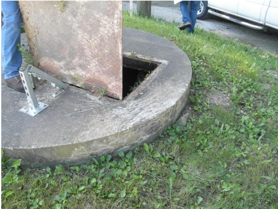
Picture T5: Map Cracked Wet Well Slab
