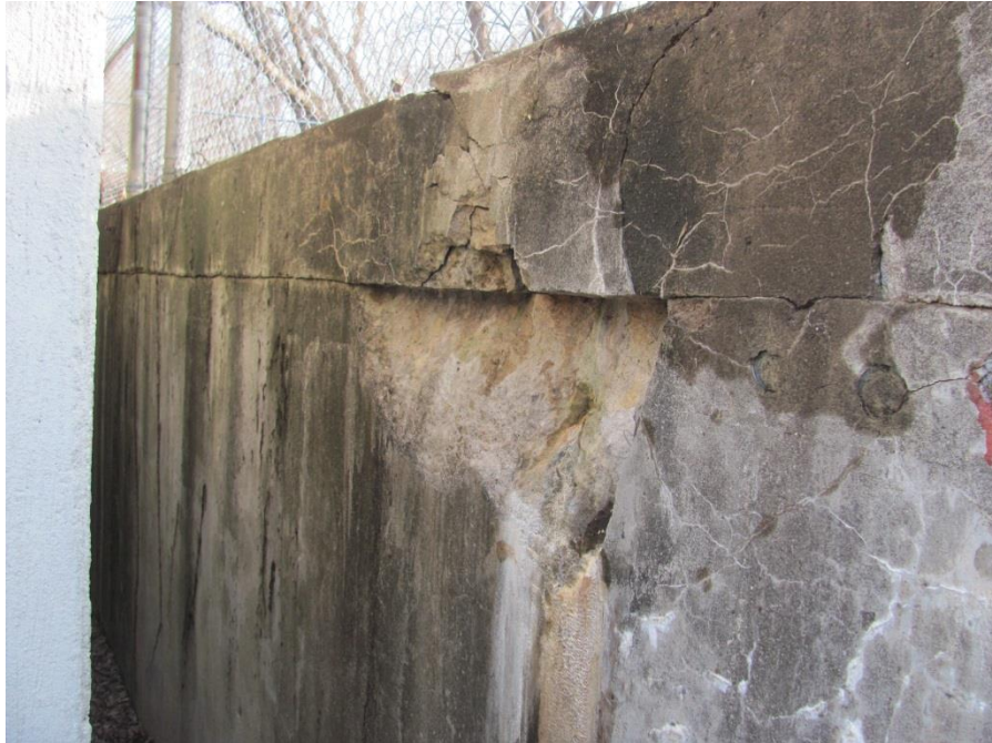
Picture NH2: Storage Tank Concrete Wall Deterioration at Slab and Top of Wall (Typ.)
