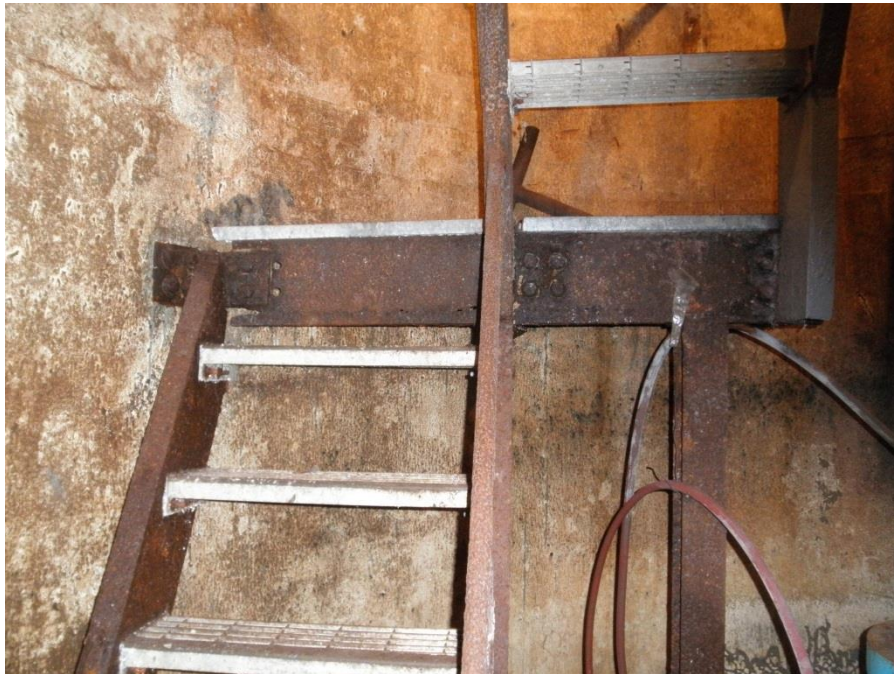
Picture CC10: Severely Corroded Channel Stairway Support
