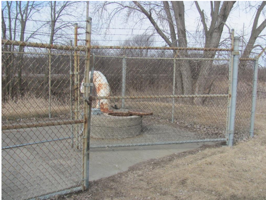
Picture H63S2: Highway 63 South Lift Station - Wet Well
