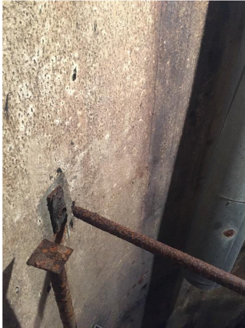
Picture CC9: Corroded Portions of the Stairway Railing System
