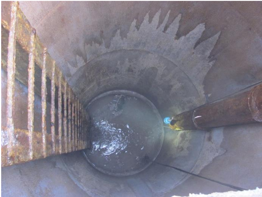
Picture T4: Wet Well Interior Showing the Unused, Inoperable Trash Basket
