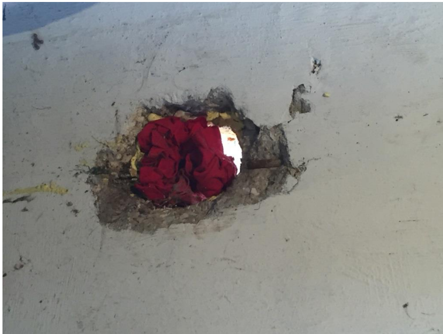
Picture D7: Inadequate Access Cover
