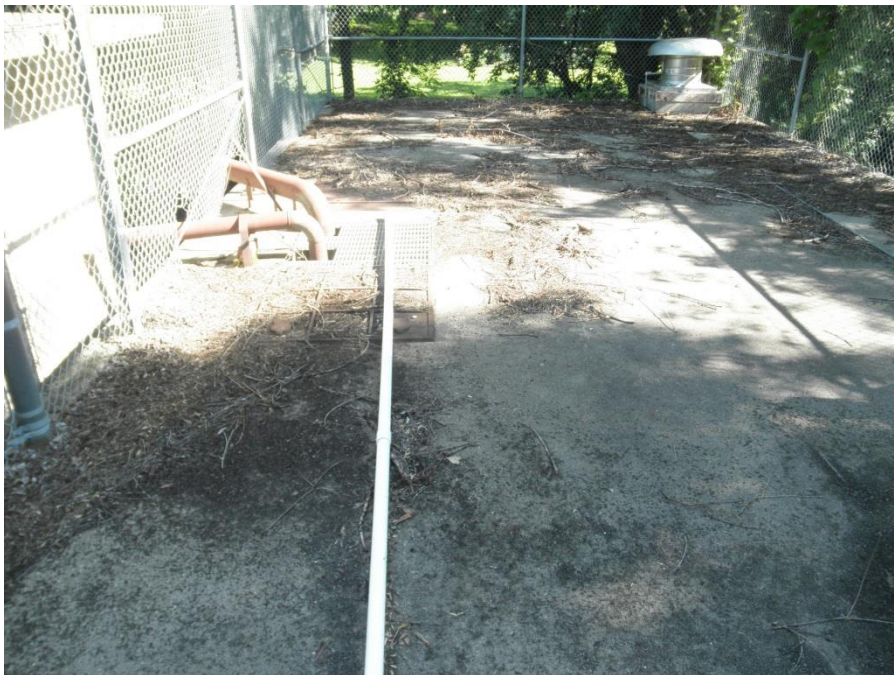
Picture NH5: Debris on Top of Slab; Note Areas of Ponding Water
