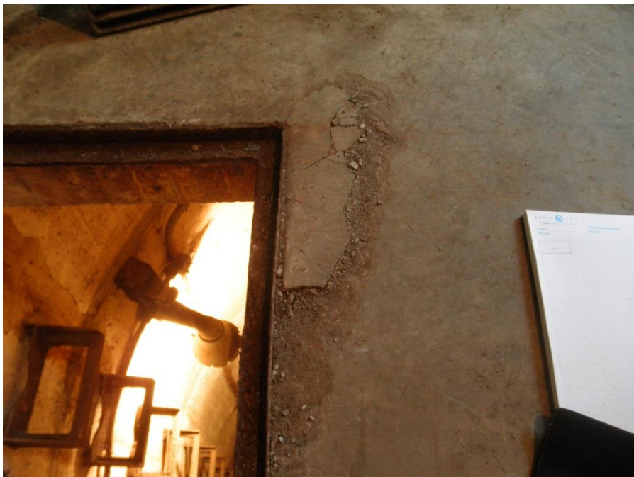
Picture T10: Spalled Concrete at Floor Access Hatch of Dry Well At-Grade Structure
