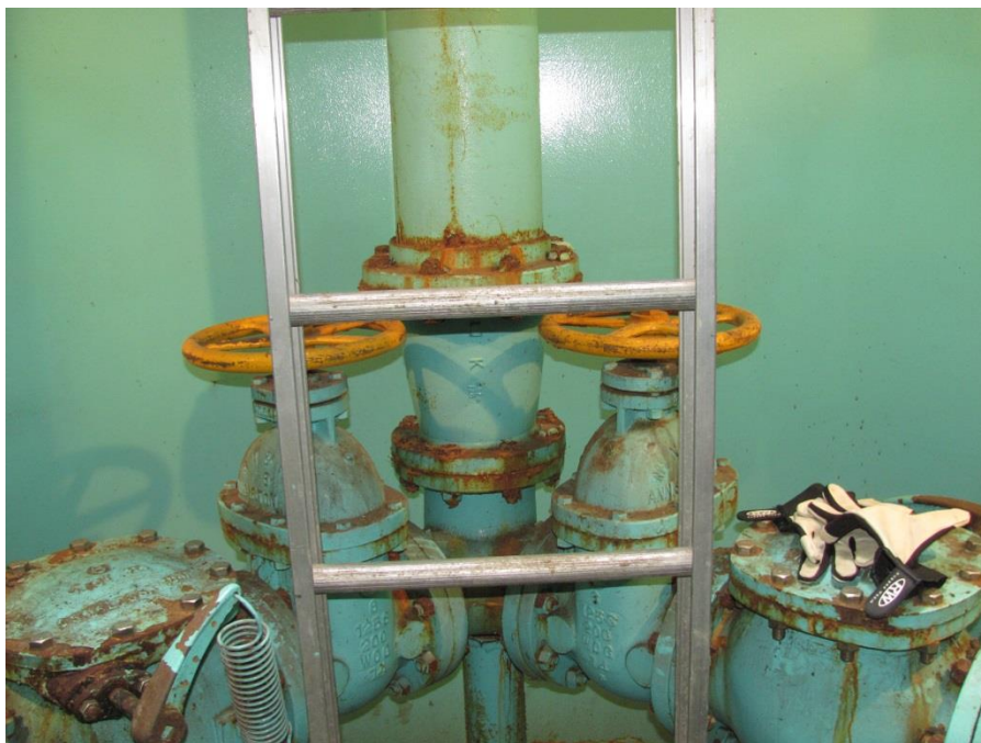
Picture H63S3: Light Corrosion of the Piping and Valves in the Dry Pit
