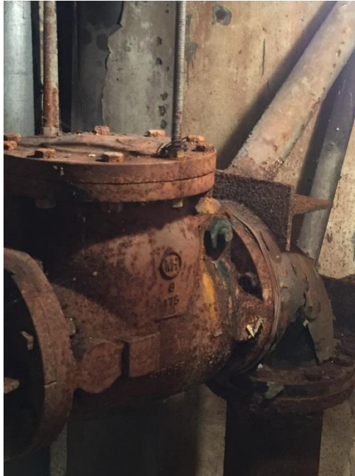
Picture CC3: Corroded Valve and Piping in Wet Well
