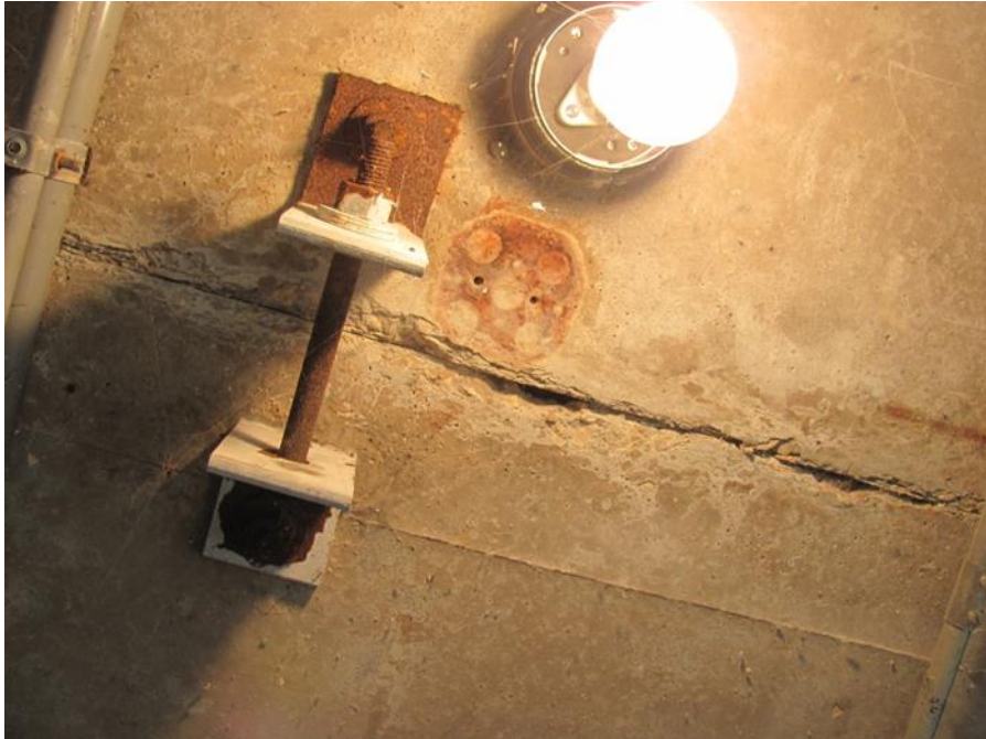
Picture T9: Minor Ceiling Slab Spalls at Dry Well At-Grade Structure Concrete Panel Joints
