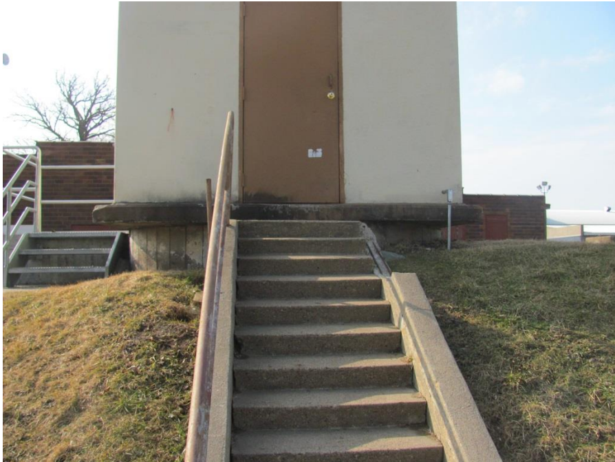
Picture CC1: Cattle Congress Lift Station; Note Damaged Access Stairs
