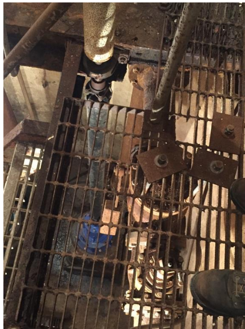
Picture CC2: Valves and Pump in Dry Pit
